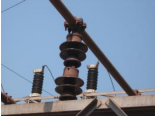
DISC AND SUPPORT INSULATOR FOR 33KV SWITCH YARD
